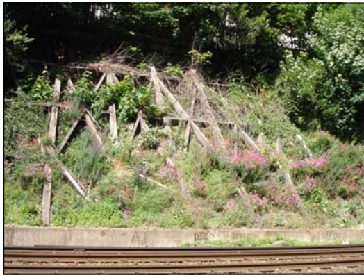
(Before: Corroding & overgrown wooden shoring)
