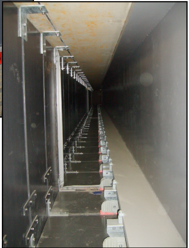
(Detail of hanger system and FRP enclosure panels fully installed on Chislehurst road bridge)
