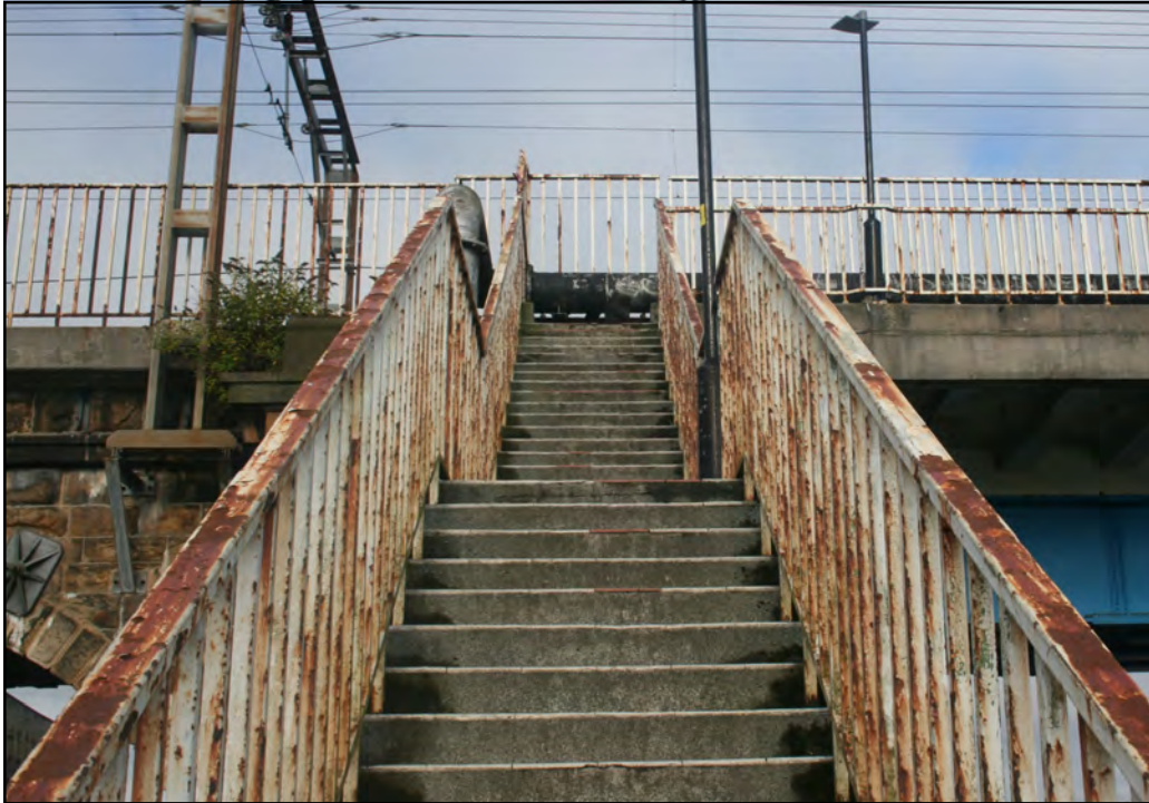
(The highly corroded stairwell before refurbishment)
