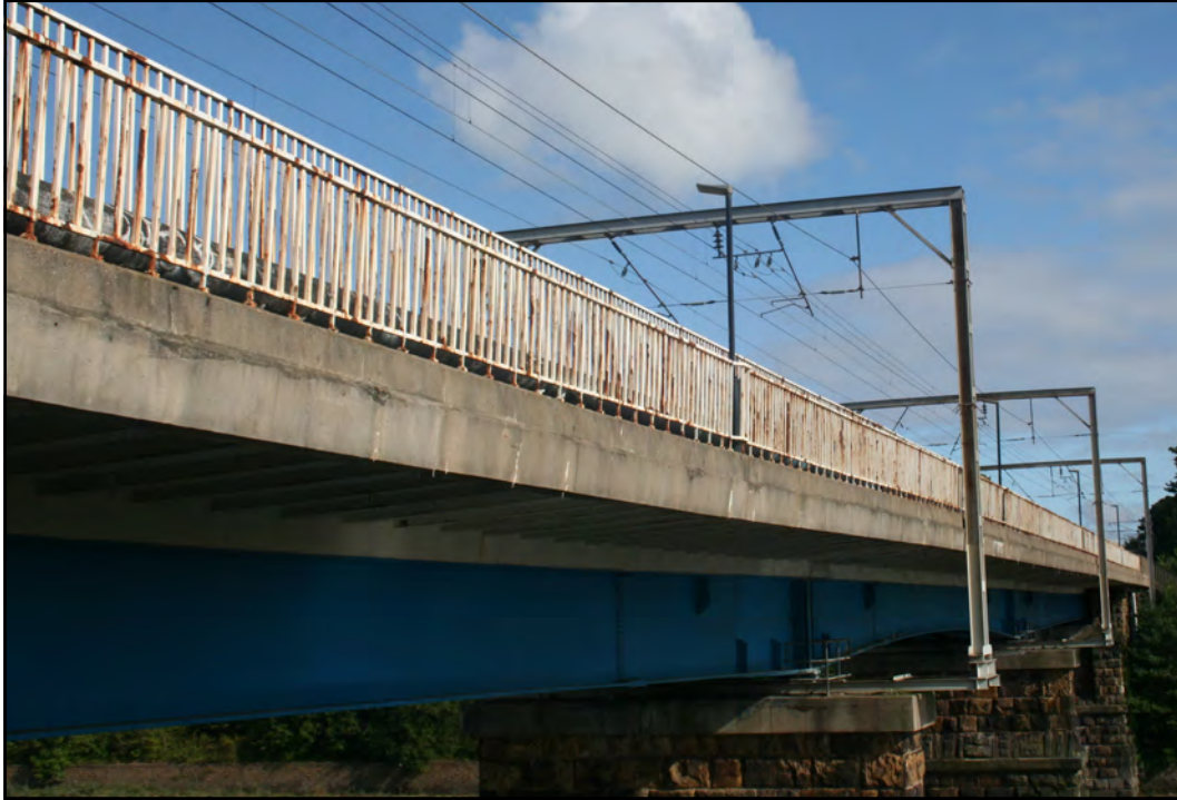
(The original steel fencing had corroded beyond repair)
