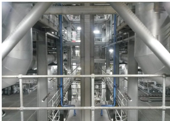
Inside Lakeside EfW, Colnbrook. Photo: Stella Job
