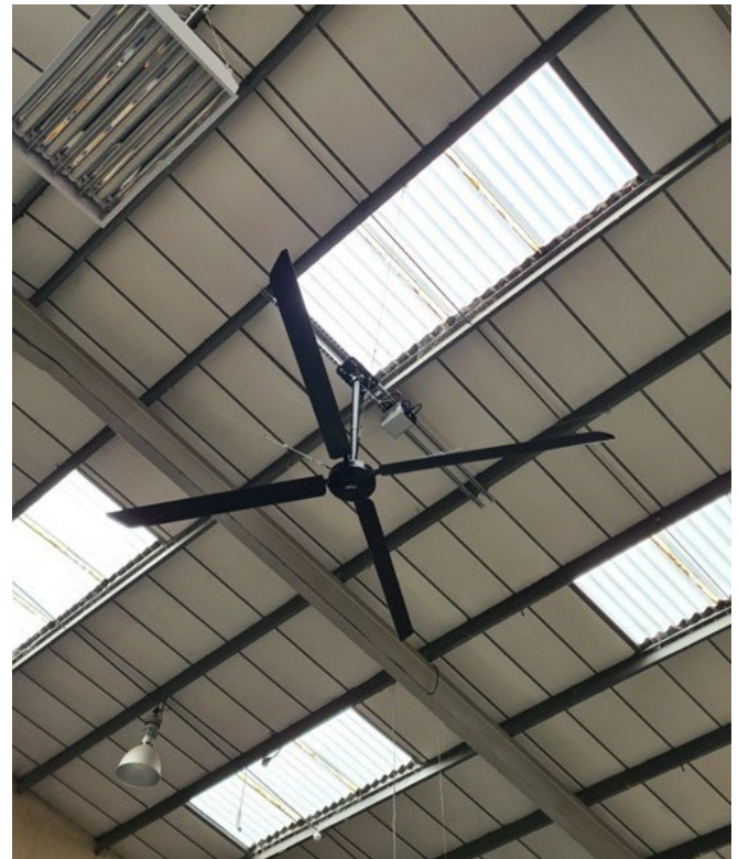
A destratification fan installed in the workshop at Far-UK is saving 2.7 tonnes of CO 2 /yr- equivalent to a year's gas use for a four bed home. Rooflights allow natural light, reducing energy demand for lighting. Photo courtesy of Far-UK.
